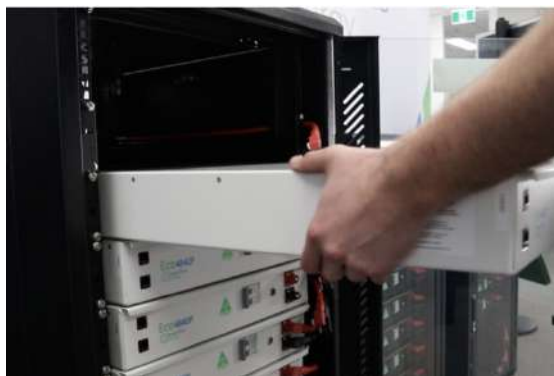
Figure 8 – Typical Battery Assembling
