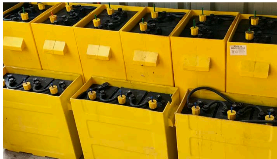
Photos courtesy of De Main Electrical (August 2019)
