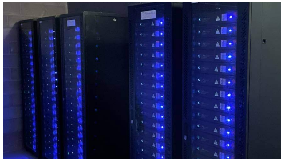
Photos courtesy of Territory Solar Solutions (May 2021)
